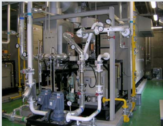
Cogeneration system that recovers waste heat and uses it to supply electricity during the daytime
