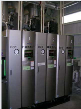
Highly-efficient boilers fueled by city gas
