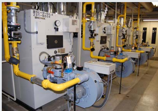
Vacuum hot water heaters (boilers) installed at the Mito Plant
