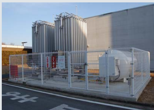
LPG supply facilities
