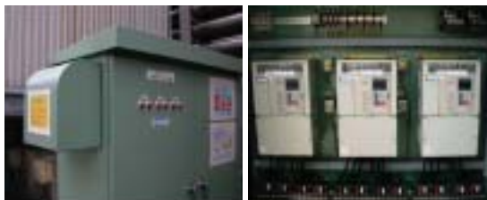
Pump inverter equipment introduced at the Kumagaya Plant
